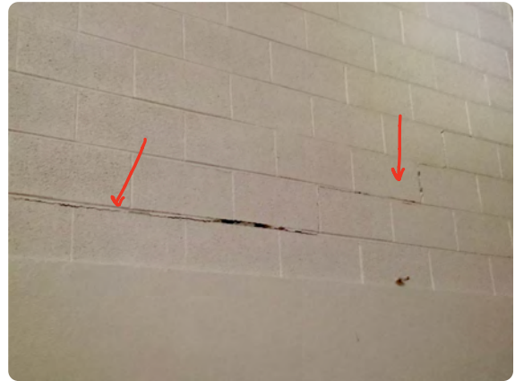
STAIR STEP CRACKS ON WALL DIVIDING MAIN GYM FROM DANCE ROOM/WRESTLING ROOM & EXERCISE ROOM.
