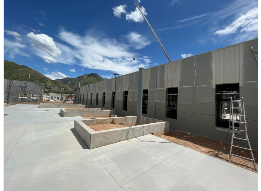
Flatwork placed in courtyard, panels for the athletics vestibule have been stood, north wall of the administration suite being painted
