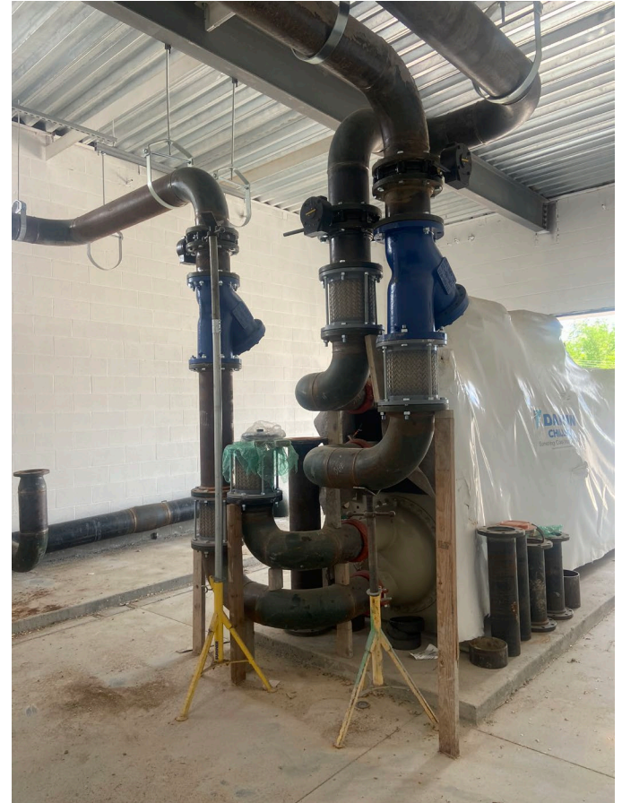
Chiller in place with piping attached
