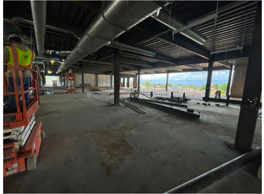
Ductwork and plumbing being installed down the level 3 corridor near general classrooms
