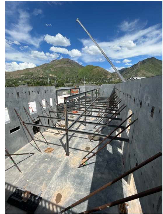
The south half administration suite panels have been stood, structural steel is being installed
