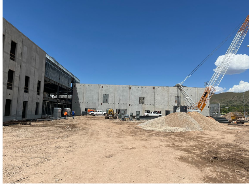
View of the administrative suite from the future courtyard, academics building on left
